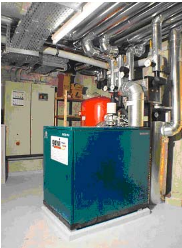
[Photo of a small CHP unit. 17 kW th .]
