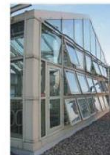
BEMS controlled windows and louvers
