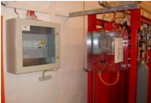
Stanice SHZ CO 2
